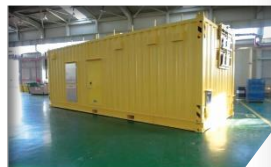
▲ ESS (Energy Storage System)
