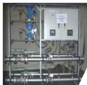
Water / Gas manifold
